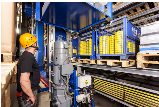
Checking the stacker cranes in the reduced-oxygen high-bay warehouse.
